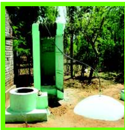
Toilet Linked Bio-gas Plant
