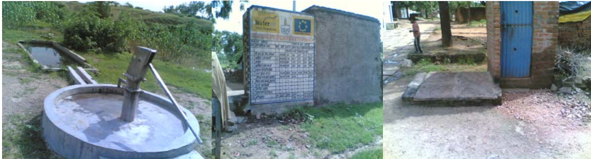
VWSC constructed new hand pump Display Board of work under taken IHHT with offset pit
