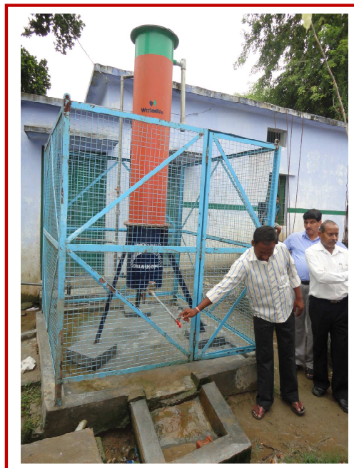
Arsenic Removal Plant (Activated alumina based)
