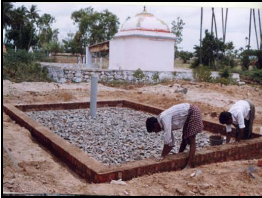
Blue metal is provided over the sand filter and a brick wall is provided so as to keep the filters and the bore well in tact.
