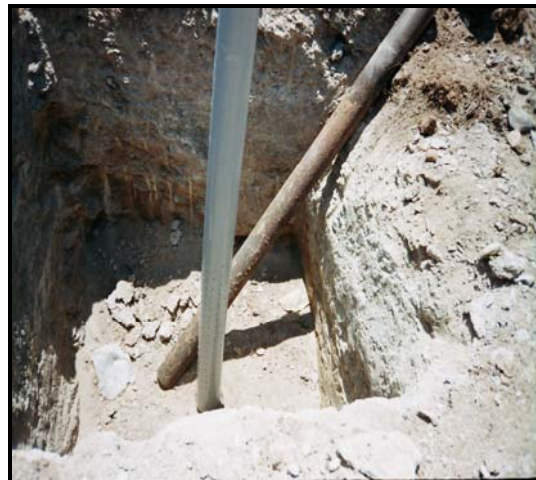
A new perforated PVC casing pipe is inserted in place of the corroded casing pipe.
