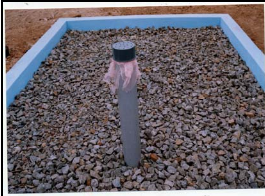
The casing pipe is wrapped up with nylon mesh and closed with an end cap that acts as an air vent.
