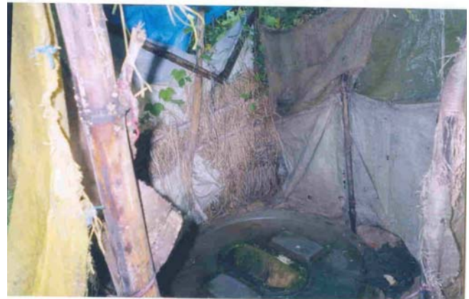
Photo: 26 Poor Maintenance of Toilet in Kultikori GP (Medinipur West)
