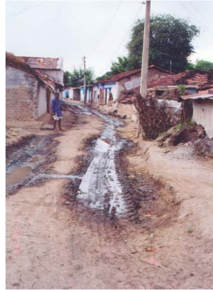
Photo: 42 Lack of proper drainage in village Kamaliya. (Sehore)
