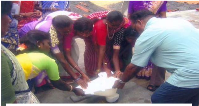
Photo: 12 Training of Women Masons to install toilet seat in Vellore District
