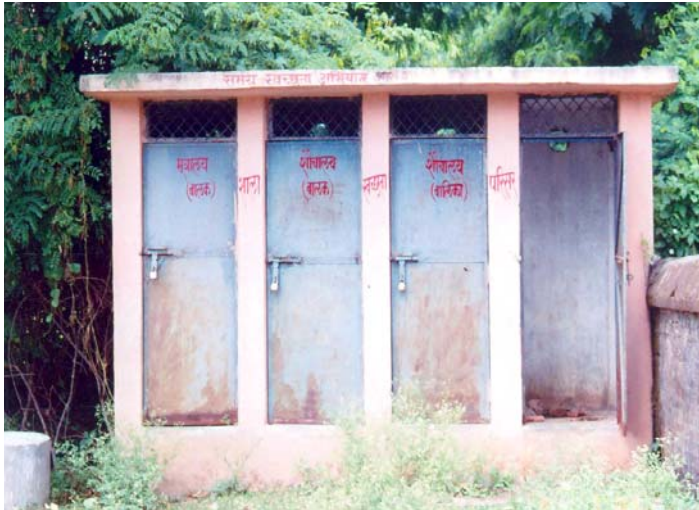
Photo: 28 School toilets found under lock and key during school hours. Water tank outside the building was filled with stones & soil. Government Primary School, Village Barha Chota. (Narsinghpur)
