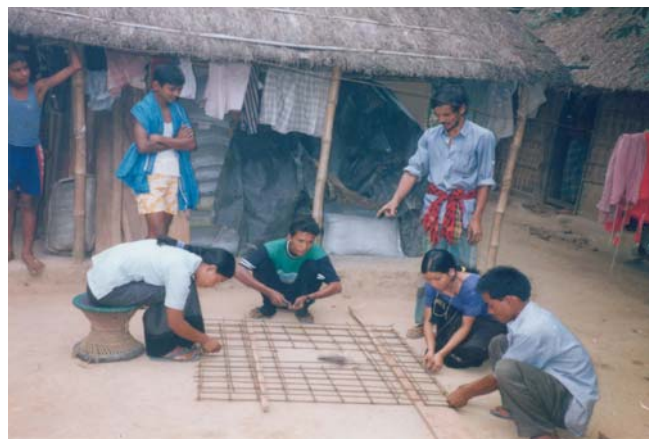
Photo: 13 PC New Gomati Village, Amarpur Block (Midnapur West); training in platform construction; women masons also being trained
